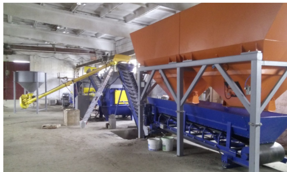
Figure 1 – General view of the technological line of Ecostroy NII-PV LLP
