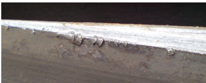
Figure 5 – VAE cross-over R-65 1/11 core burst at the yard station
