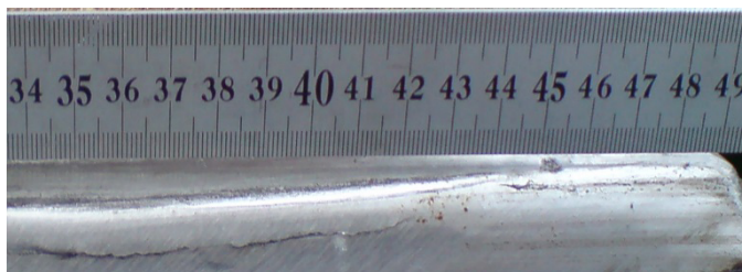
Figure 14 – VAE cross 60E1 1/11 core longitudinal crack at Carozas station
