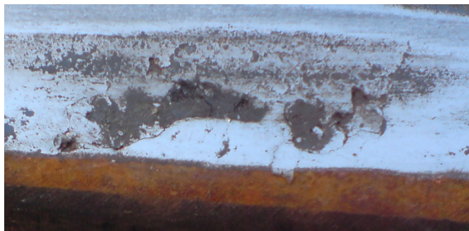
Figure 8 – VAE cross 60E1 1/11 cracks at Slampes station
