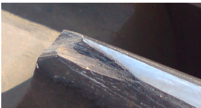
Figure 6 – Breakage of the end of the core of VAE cross R-65 1/9 at the Skirotavas station
